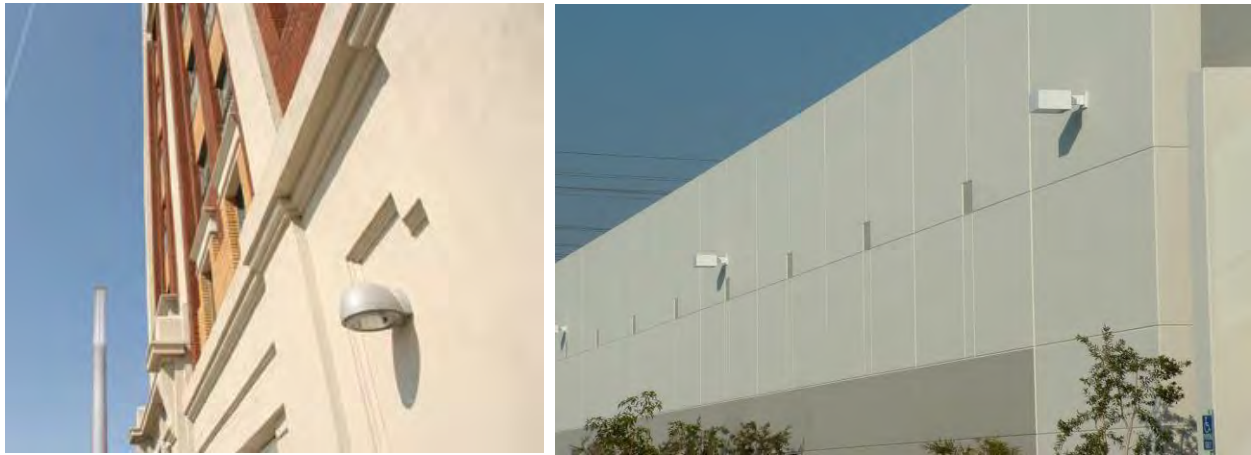
Lighting Fixtures Shield
