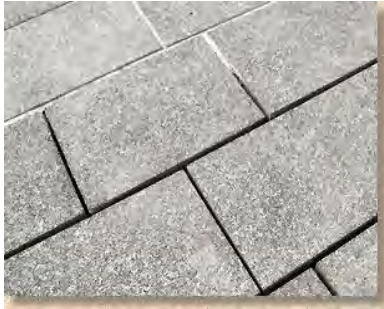
Open Jointed Surface
