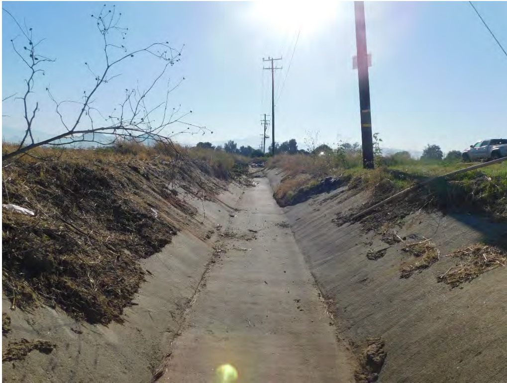
Photograph 7: From the culvert, looking east at the paved portion of the road-side ditch that conveys flows to the east.
