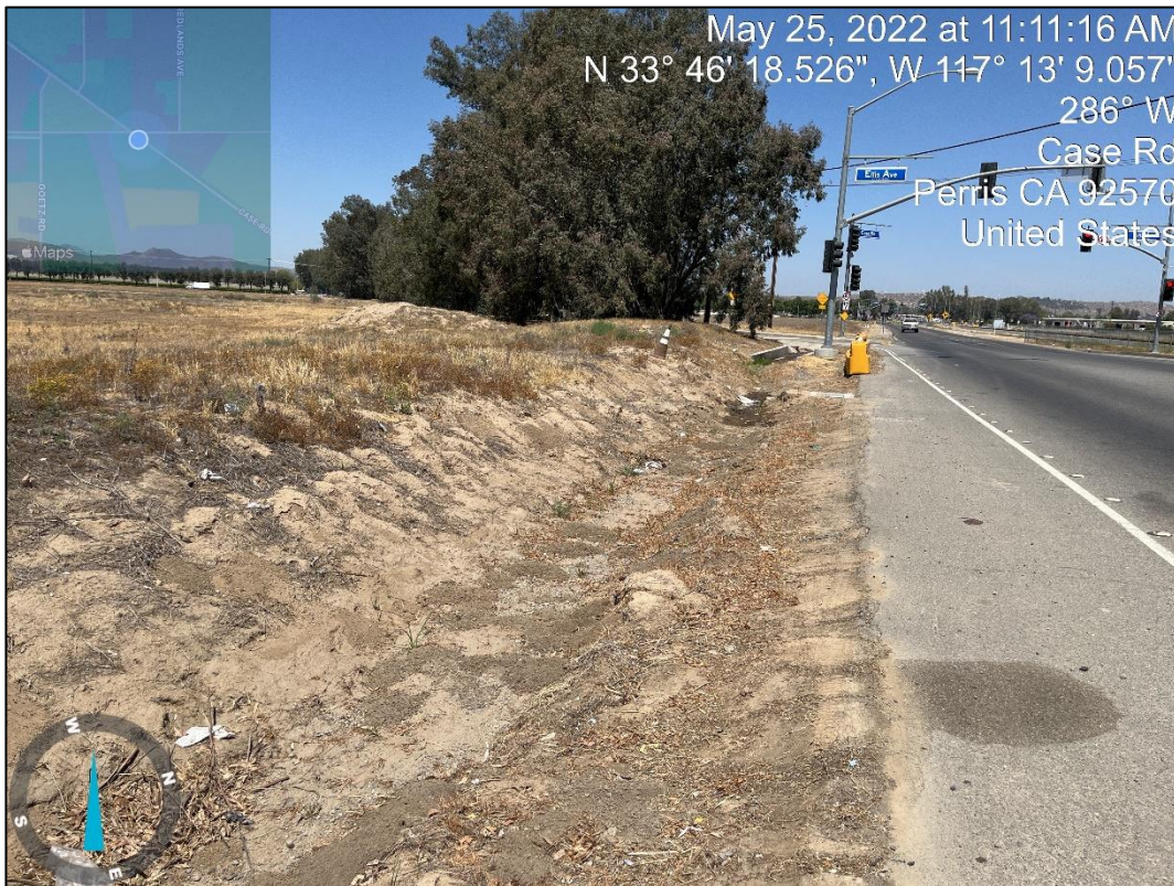
The ditch changes from concrete lined to natural bottom along Case Road.
