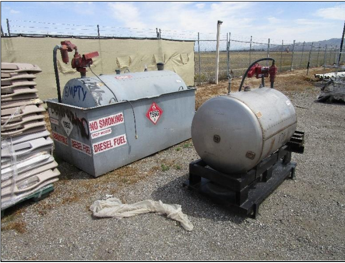
19. Diesel fuel storage tank and vicinity on north central side of Subject Property.
