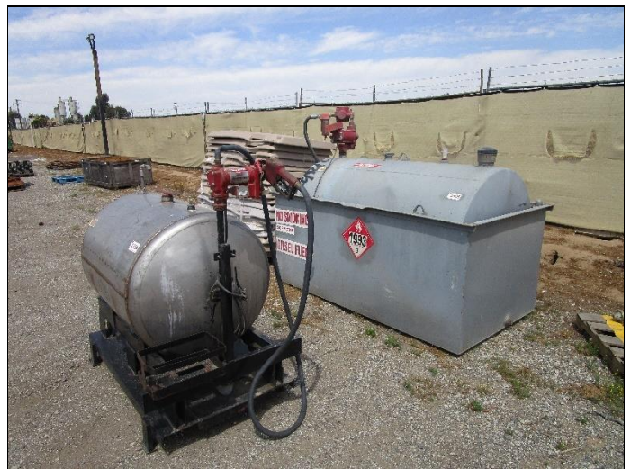
18. Diesel fuel storage tanks on north central side of Subject Property.
