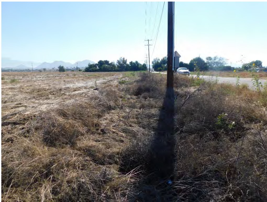
Photograph 8: Looking east at the roadside ditch that conveys flows along Orange Avenue, just east of the paved portion of the ditch.
