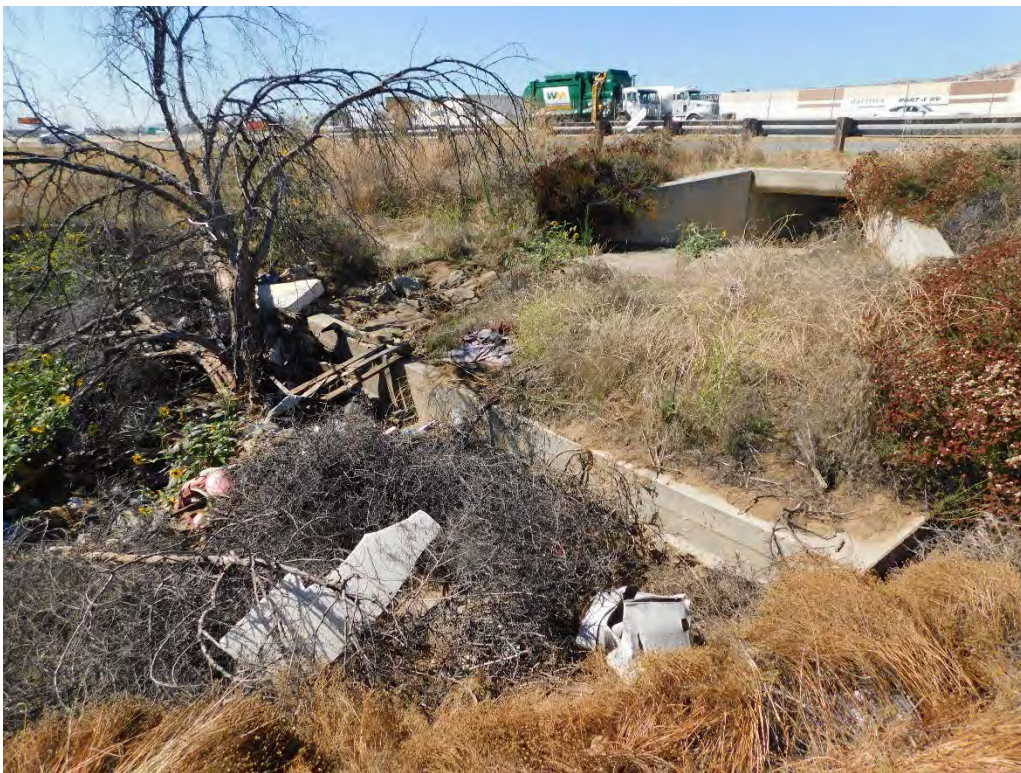
Photograph 2: From the northern banks of Drainage 1, looking southwest at a paved box culvert and stepped spillway that convey flows east through the project site.
