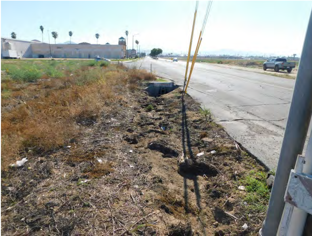
Photograph 11: Looking east toward a culvert which conveys flows under Barrett Avenue to the east of the project site.
