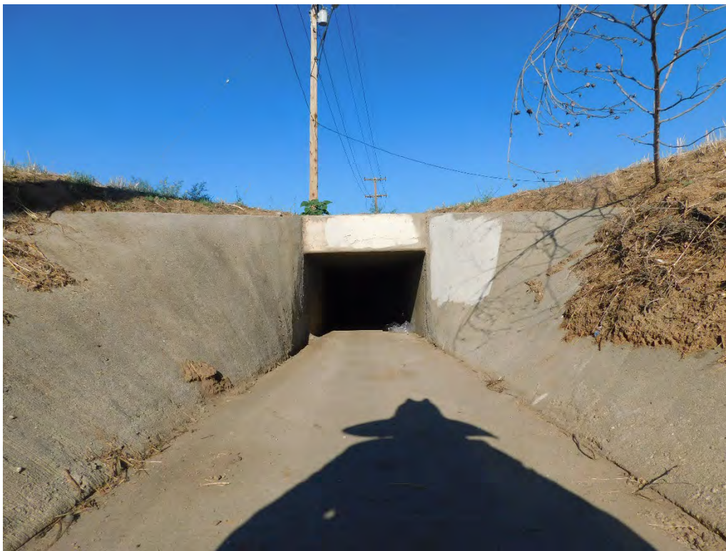
Photograph 6: Looking at the culvert that conveys flows from the west along Orange Avenue.
