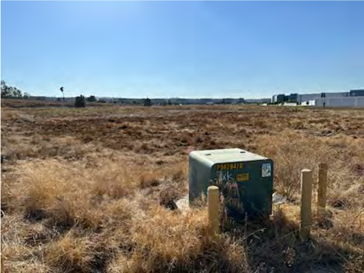
Pad-mounted transformer located in the center of the site along Nevada Road.
