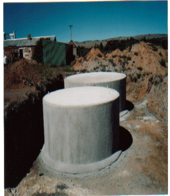
Figure B: Large Scale Capture and Use Tank
