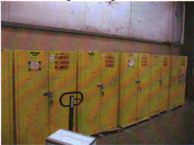
Flammable materials storage
