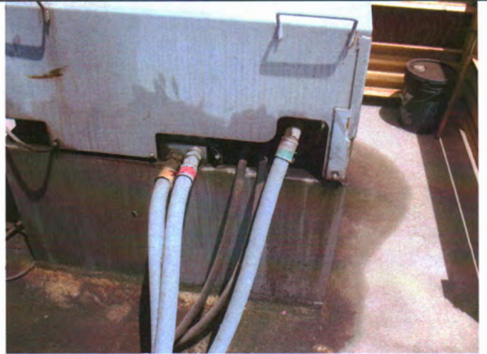
Old hydraulic leak from trash crusher
