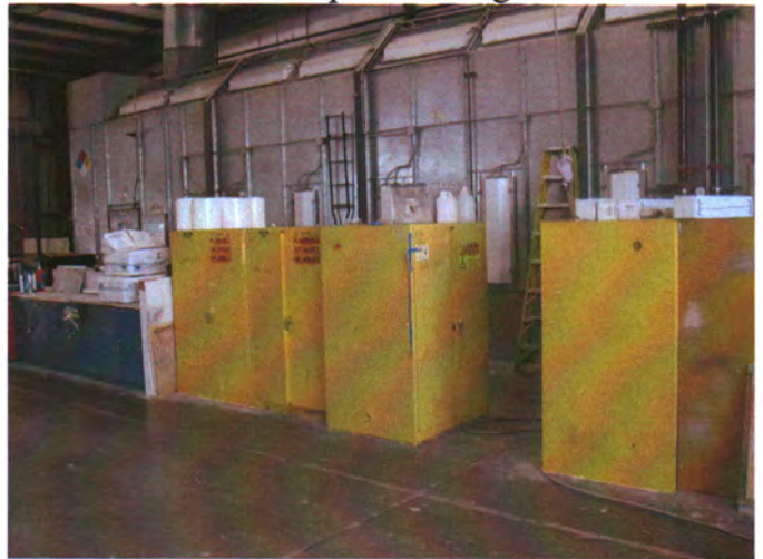
Service Center flammable storage
