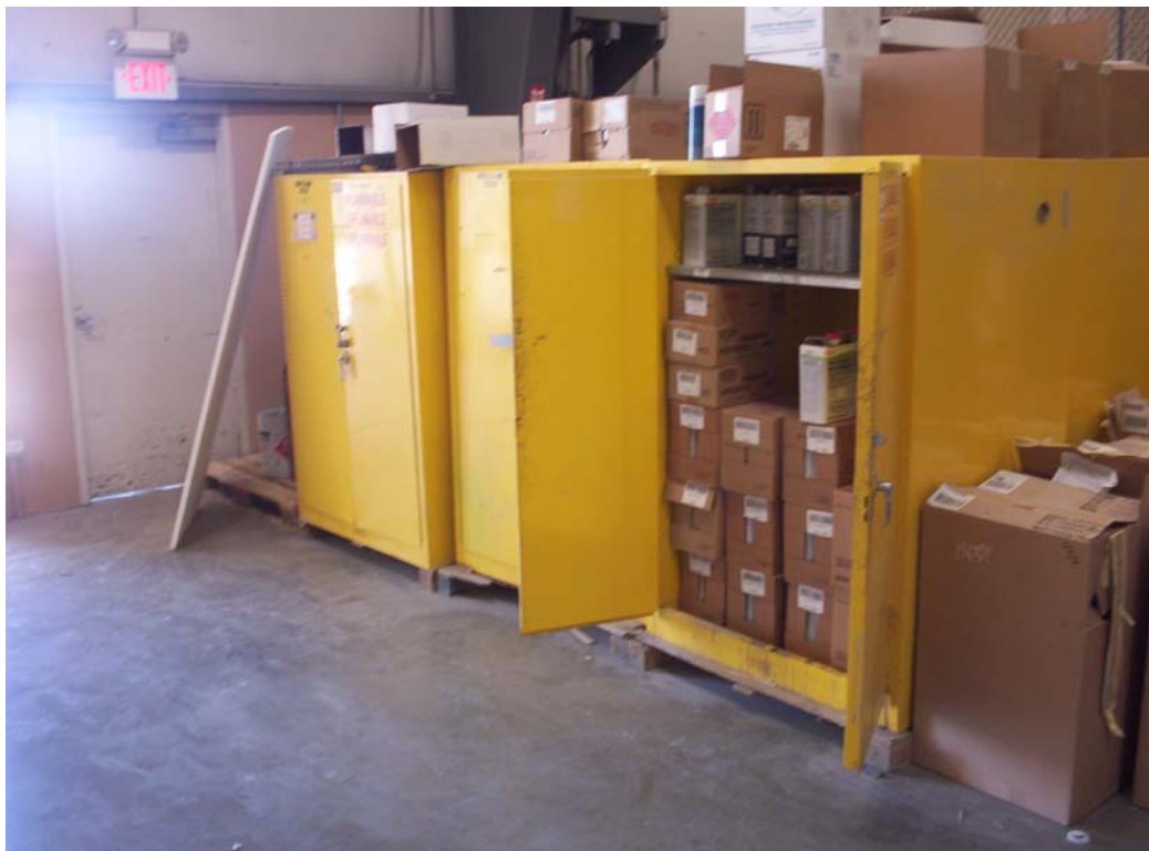
Photo #24: Typical hazardous materials storage cabinets.
