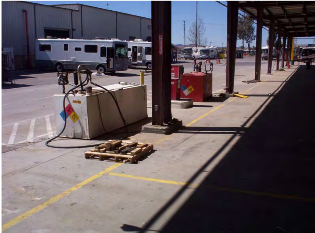
Photo #5: Aboveground diesel fuel tanks adjacent to Building 1.
