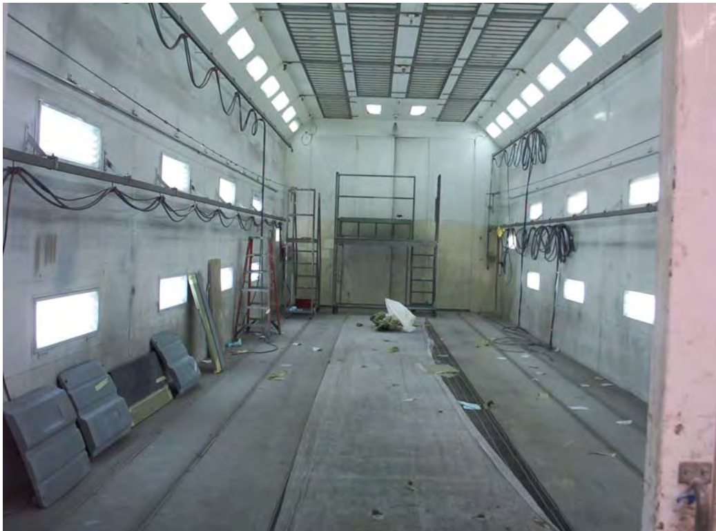
Photo #14: Typical paint booth within Building 5.
