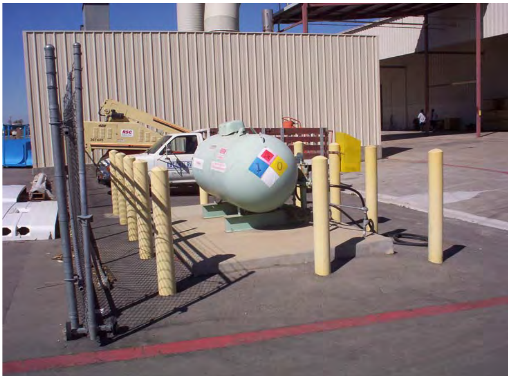
Photo #10: Propane AST at the northeast corner of Building 4.
