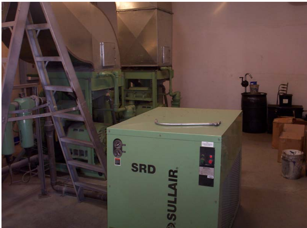
Photo #18: Compressor room within Building 5. A drum of compressor oil is visible.
