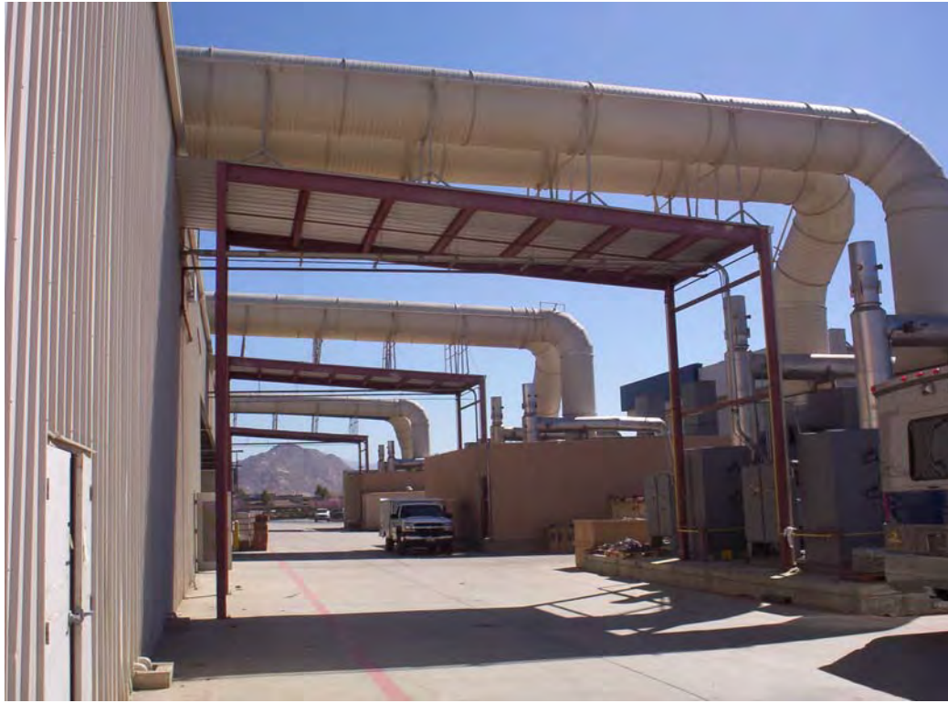
Photo #17: Air handlers connected to Building 5 (southern side).
