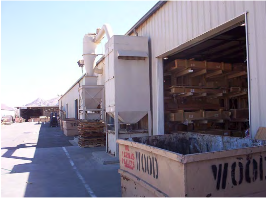
Photo #3: Northern edge of Building 1 (3411 N. Perris Boulevard). A dust suppression system is visible. Building 3 is visible in the background.
