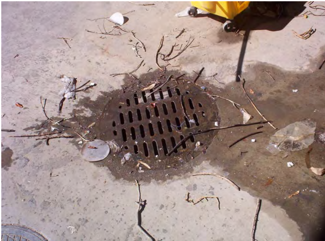
Photo #16: Manhole above a clarifier along the southern edge of Building 5. The clarifier is associated with the rain test area (Photo #15) and leads to two underground water tanks.
