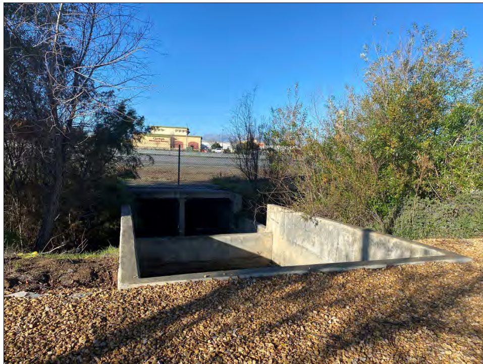
Photo 12. View of the storm drain (non-jurisdictional) and associated vegetation located at the western end of Illinois Avenue within the Project Footprint; facing west.
