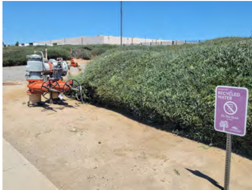
Water pump located south of the subject property along Morgan St
