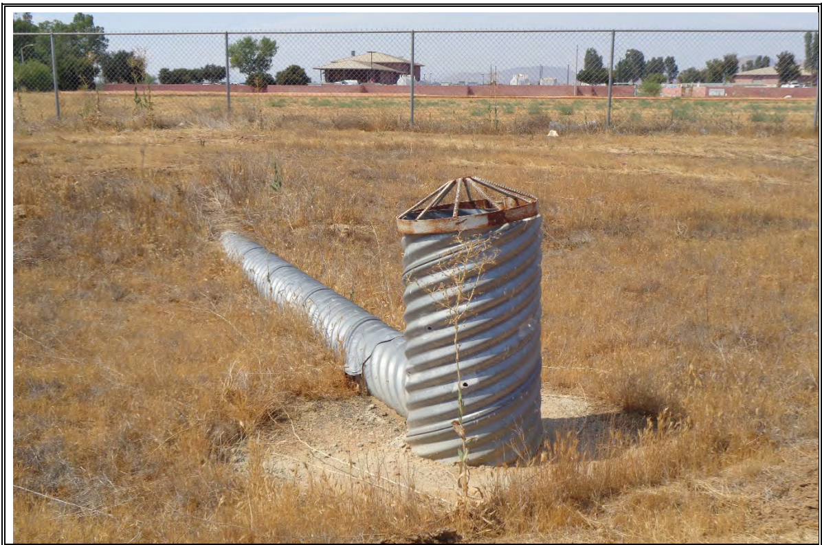
Photograph Number 10: View of catch basin located in the middle of the property.
