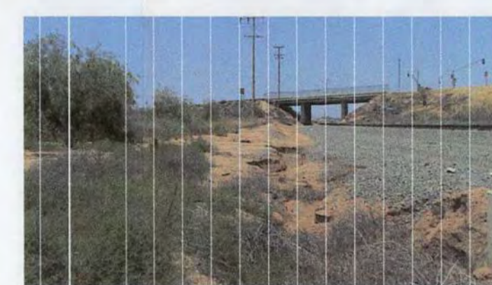
#14 - EROSION AT DOUBLE 36IN PIPE FACING NORTH
