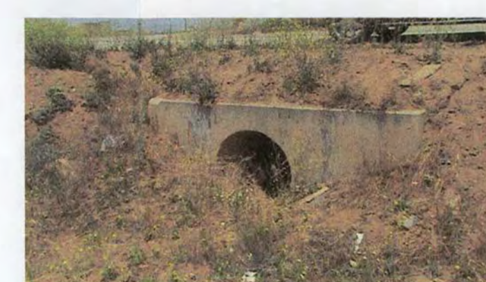
#18 - SINGLE 42IN PIPE CROSSING HARVILL AVE FACING NORTH EAST
