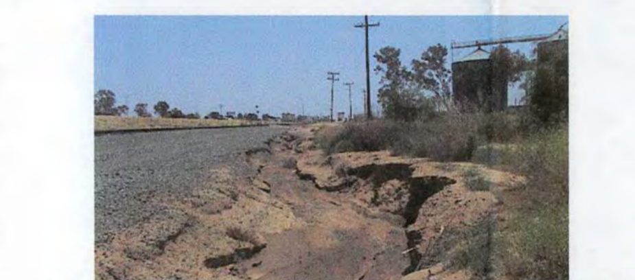
#15 - EROSION AT DOUBLE 36IN PIPE FACING SOUTH
