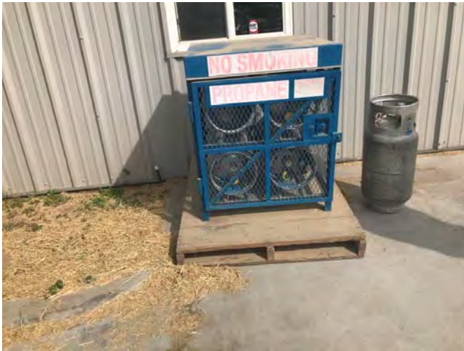
7. Propane fuel tanks.
