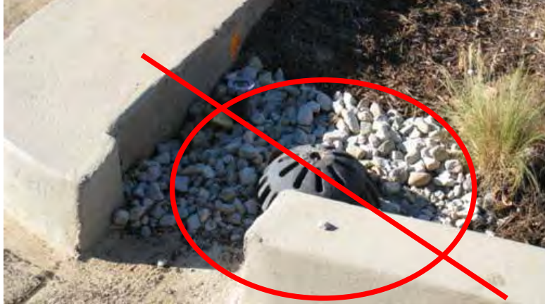
Figure 6: Incorrect Placement of an Overflow Inlet.
